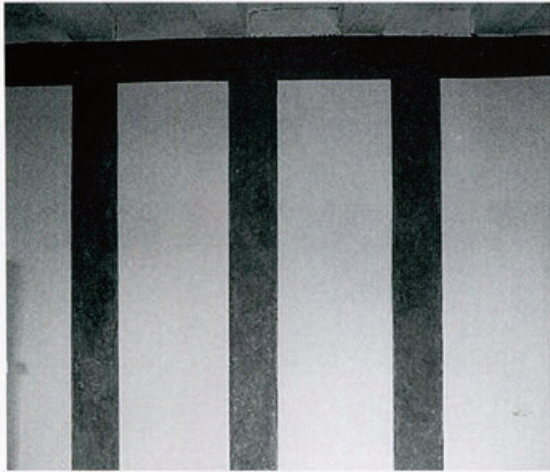
Fig. 9: Fictive painted grey studs at the back of the partitions of the two North rooms in the East Wing
