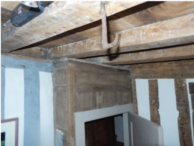
Fig. 6: Back parlour room. The 1630 paneled portal has a larger 19th c door than the original. The width of the upper cornice is indicated by a change in the timber colour. Originally this was set off by a plastered ceiling with painted studs on both sides. One of four old food hooks is shown, positioned over the 19th century stairs to a cellar. This was probably taken from the old kitchen ceiling.
