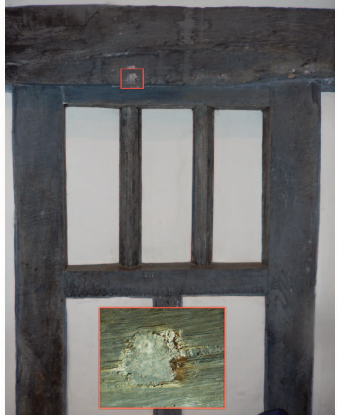
Fig. 11: The 1630 former 'room between the doors' has a plastered-covered peg hole that retains the original grey colour. The studs are painted to match, but the original oil-bound black pigment on the mullions was to give the illusion of dark stone.
