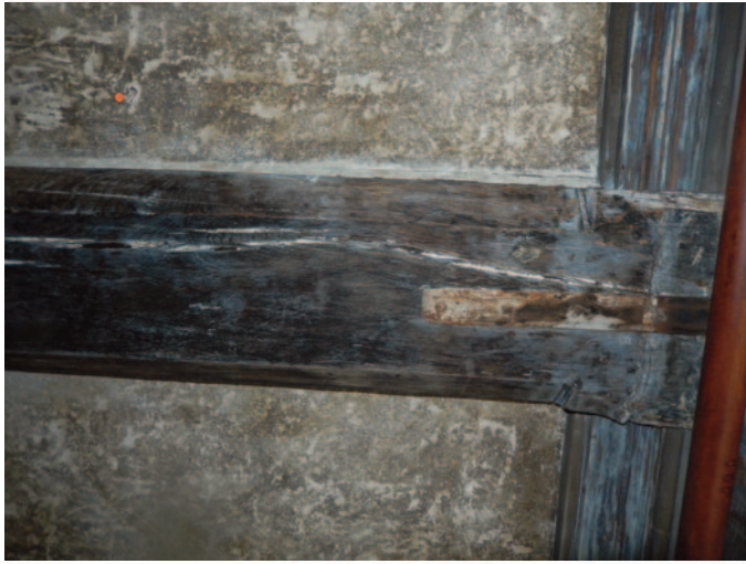
Fig. 7: Kitchen, 1620. A gap between the painted plaster and bridging beam was caused by the timber shrinkage of the beam. This has historic unpainted infill plaster, proving the painted plaster was intentional and original.
